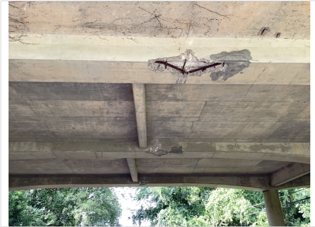
Collision damage to beams in span #2
