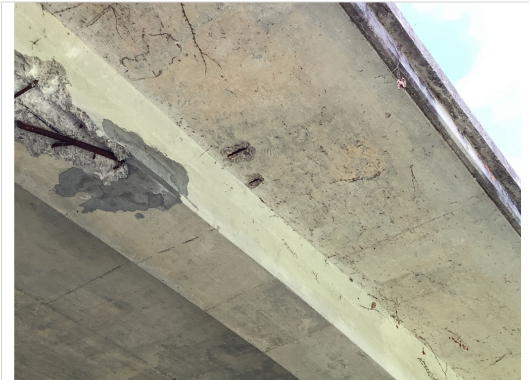
Typical spall in overhang
